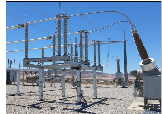
161 kV Current Transformers
