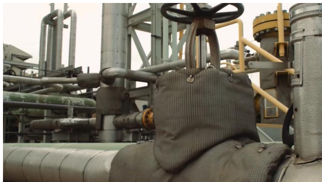
Components wrapped in fire-retardant material to protect susceptible components against freezing during winter months.
