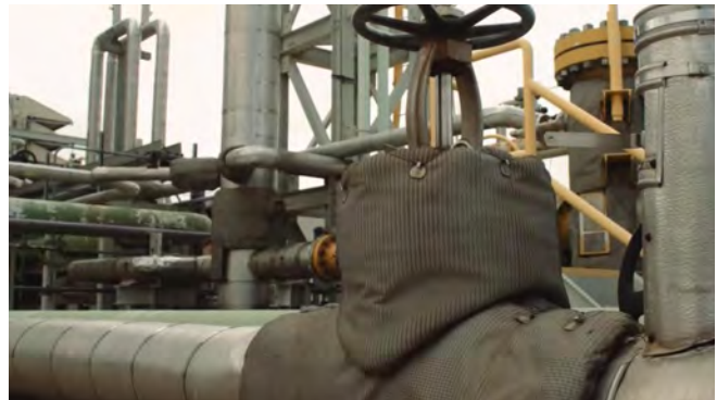
Components wrapped in fire-retardant material to protect susceptible components against freezing during winter months.
